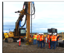
Workers with small business Hayward Baker, Inc. injected cement-based grout into 21 buried waste locations to stop rain and snow melt from infiltrating the contaminated waste produced during historic operations at the Idaho site.
