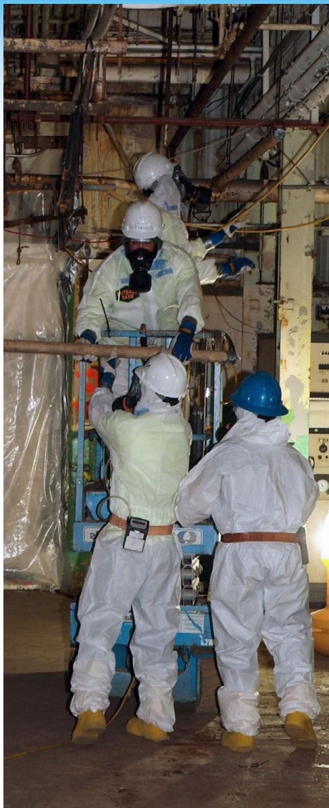
Recovery Act workers remove asbestos from the C-410 Feed Plant to prepare it for demolition in late 2011 or early 2012.
