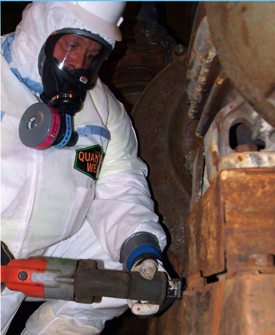
A Recovery Act worker saws a bolt loose so that a motor can be removed from the Feed Plant, which operated from 1957 to 1977. Uranium hexafluoride and fluorine were manufactured there.
